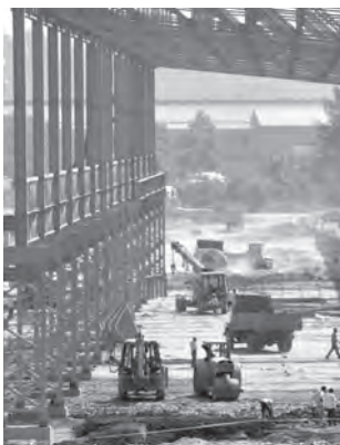
Stainless Steel Plant for Viraj
